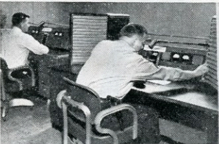
Two easy-to-operate consoles route calls to fire and police apparatus all over Philadelphia.
